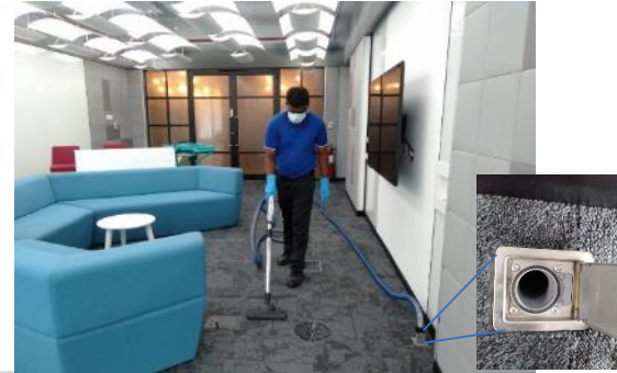
Centralized Vacuum System
